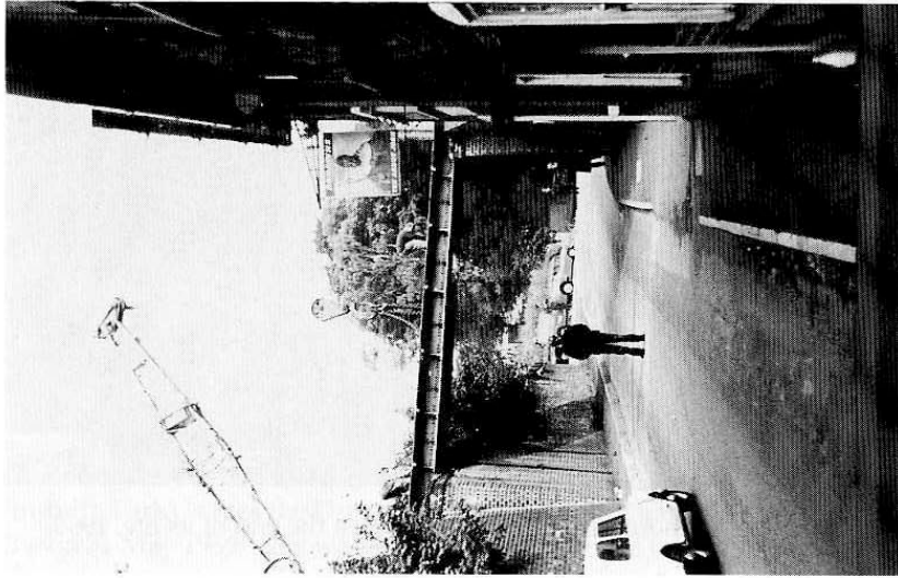
32 Ready for lift-off! The final moments of the railway bridge. (Courtesy, Barry Wood)
